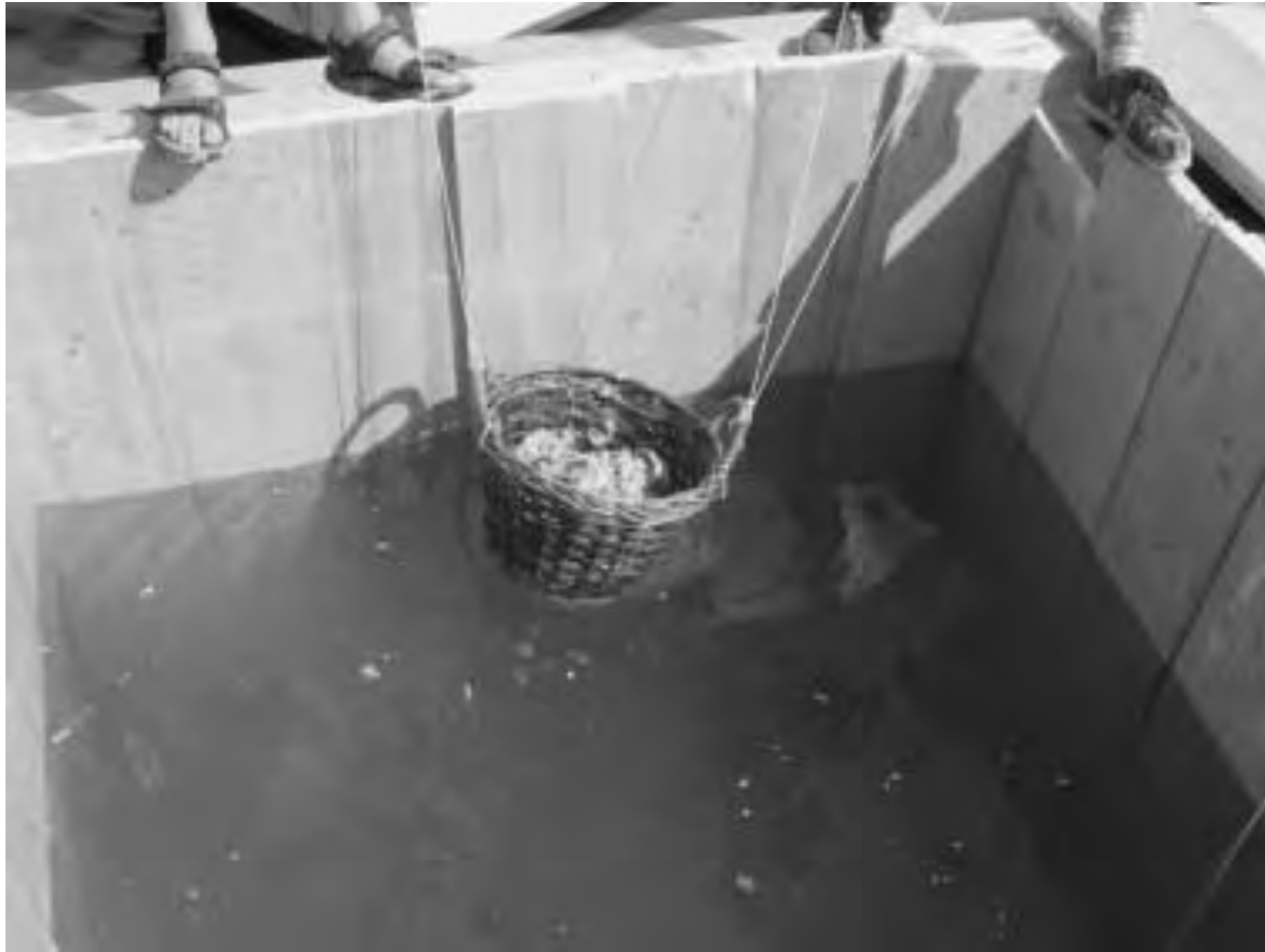
Figure 2. Mortar is lowered into the form using a wicker basket with two drop lines along with a trip line. (R. L. Hohlfelder)
