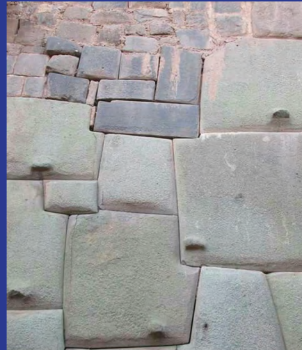
No gap in between
