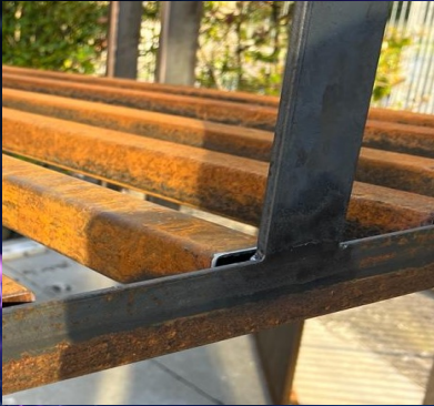
UNTREATED RUST METAL
