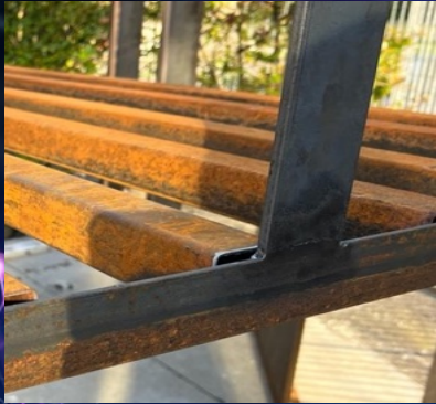
UNTREATED RUST METAL
